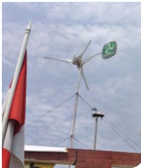
2kWh wind turbine installed on the roof of Media Centre
